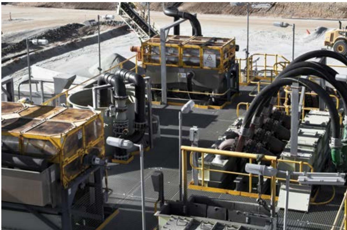
A lithium mine processing plant Western Australia, Australia.
