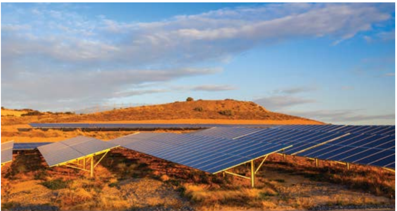
Solar farm, South Australia, Australia.
